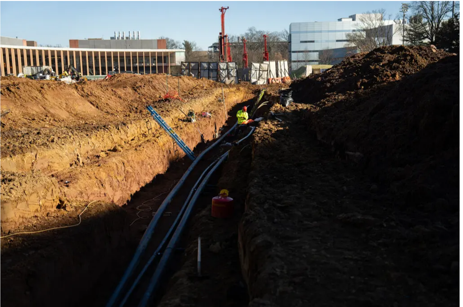
Pipes at one of the well sites on the campus. Maansi Srivastava/The New York Times
