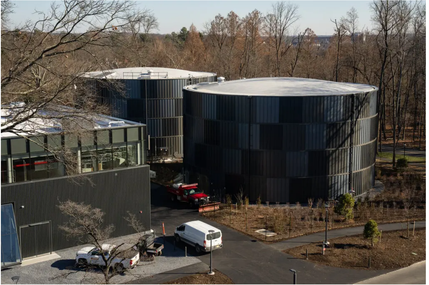
The system's water tanks, one for hot water, the other cold, each holds 2.2 million gallons. Maansi Srivastava/The New York Times
