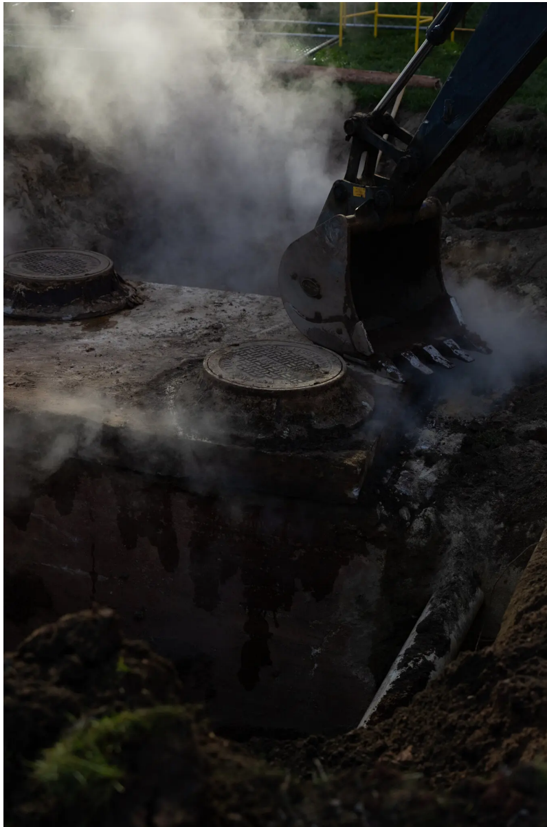
An old steam system site that is being decommissioned. Maansi Srivastava/The New York Times
